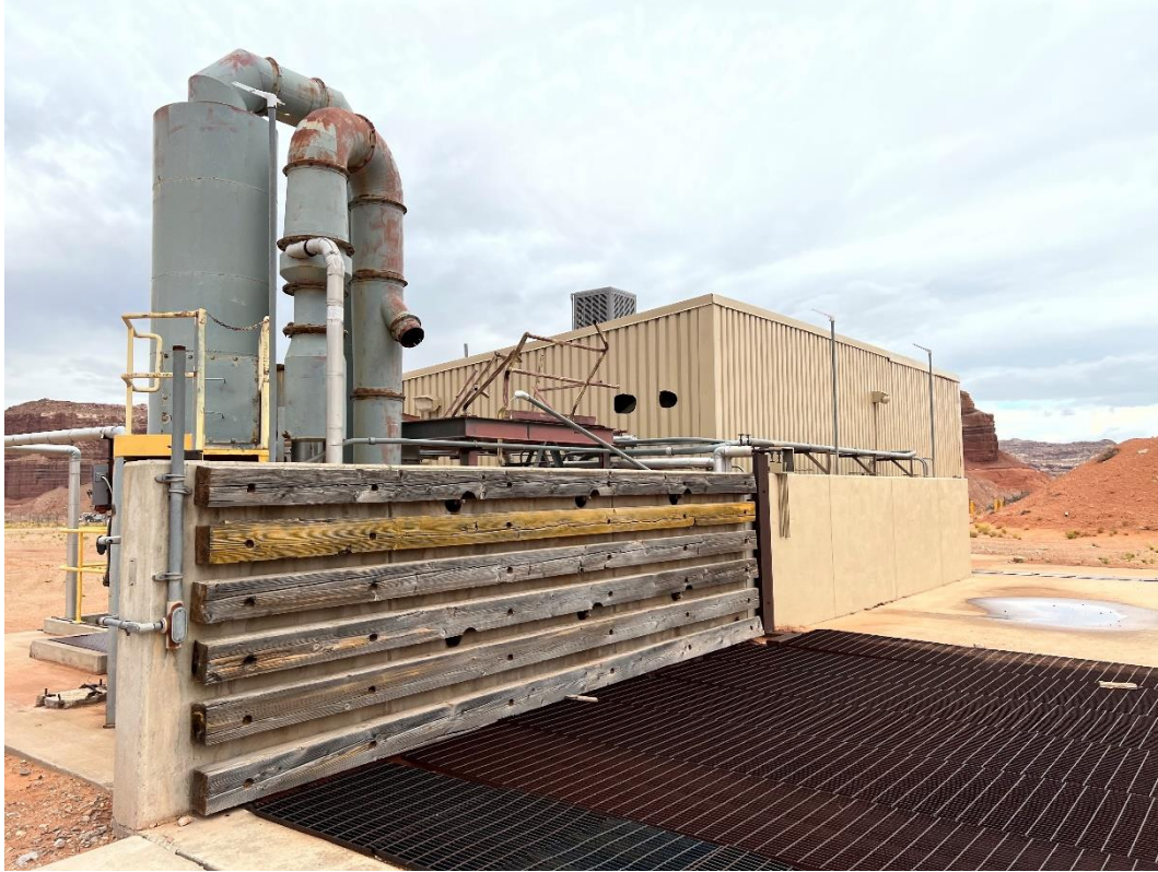
Figure 2: Shootaring Canyon Mill – Upper: above ground at the run of mine ore feed drop point for haulage trucks. Lower: underground immediately below ore drop showing RoM ore feed-to-conveyor
