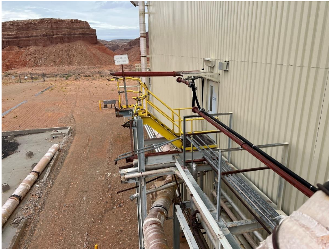
Figure 7: CCD Circuit Site – Upper: view of exterior of building housing leaching circuits where CCD circuit previously connected to the system; Lower: remnants of dismantled/removed CCD circuit site – reconstructed CCD circuit will go here
