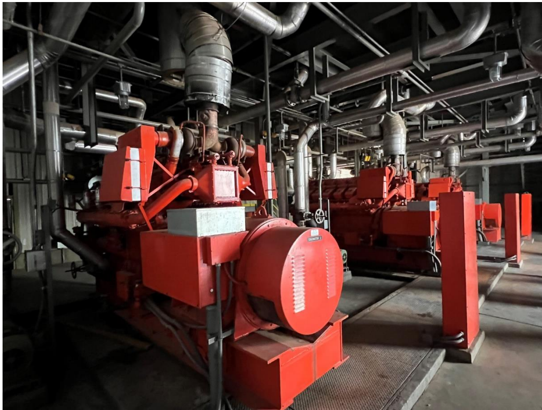
Figure 11: Upper: inside the powerhouse of the mill – the lightly used gensets will need replacing to meet modern emissions standards. Lower: Warehouse facilities
